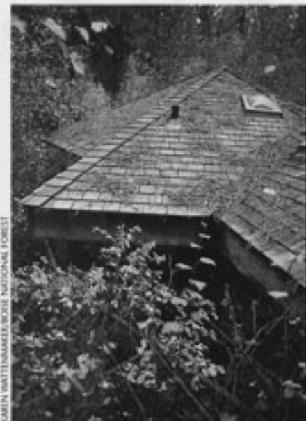
Conifer needles on roofs are one of many fire hazards that can be avoided.
